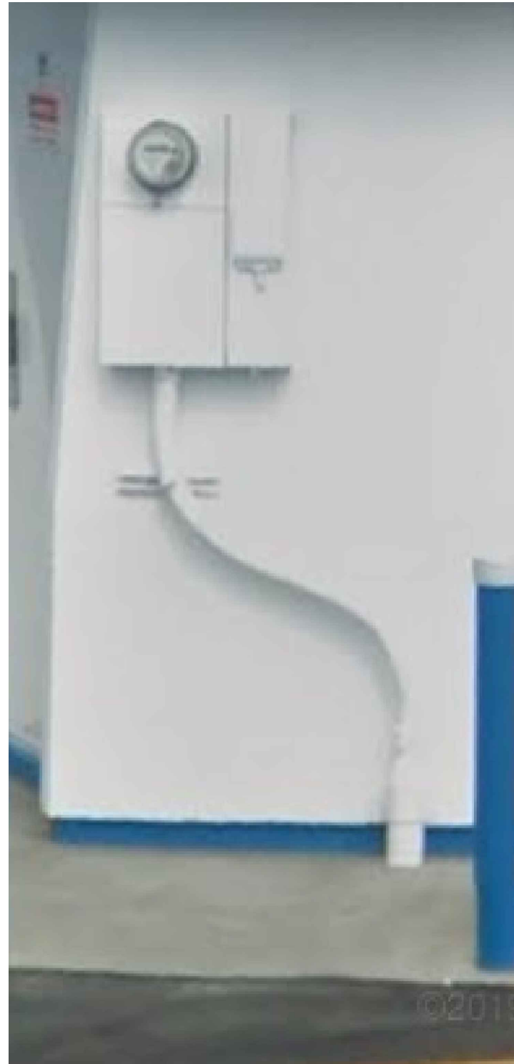
5 PHOTO - EXISTING METER SCALE: NTS
