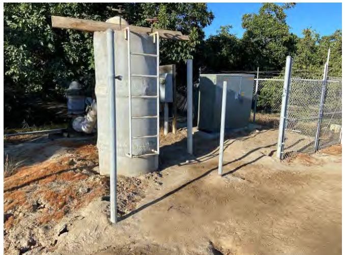
4. Transformer, irrigation well, and standpipe on north portion of Subject Property.
