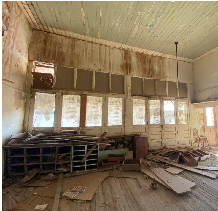
VIEW OF SOUTH WALL FROM INTERIOR WITH LARGE STOREFRONT NEEDING SEISMIC REVIEW
