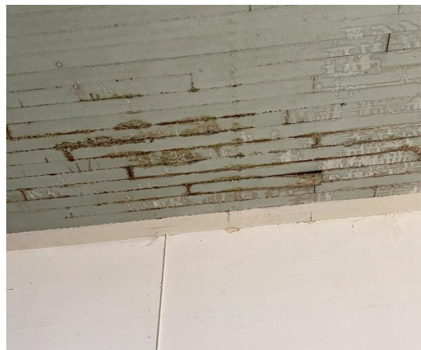
VISIBLE WATER INTRUSION AT ROOF
