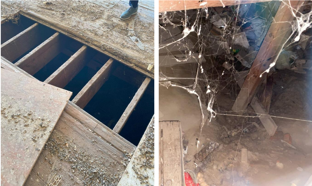
CONDITION OF FLOOR FRAMING AND SUB-FLOOR POST WITH SETTLEMENT
