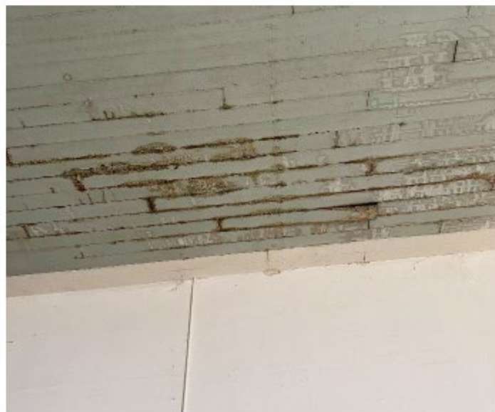
VISIBLE WATER INTRUSION AT ROOF
