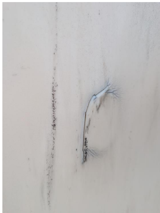
Stress fracture that became a crack
