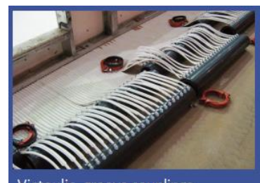
Victaulic groove couplings make for quick and easy connections between main header sections.
