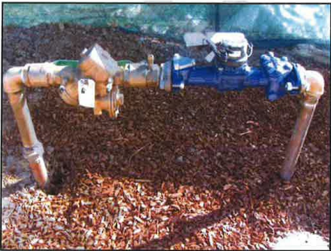
Backflow Preventer (Park Strip)
