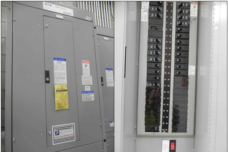
EXISTING HOUSE PANEL
