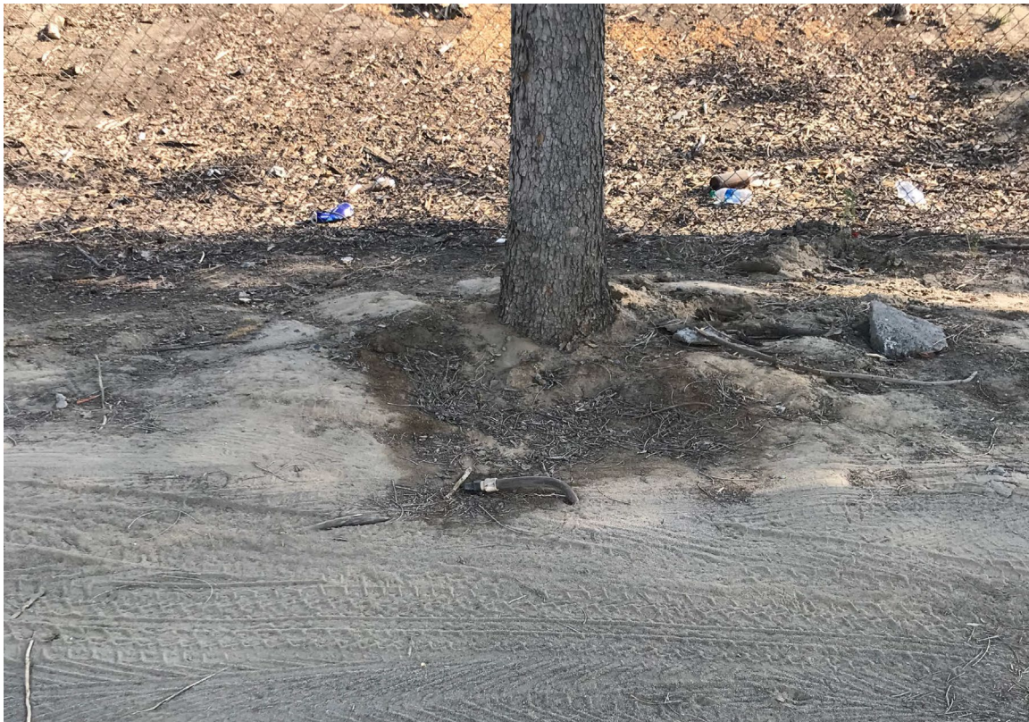
Broken city irrigation sprinkler head due to vehicles driving over sprinklers.
