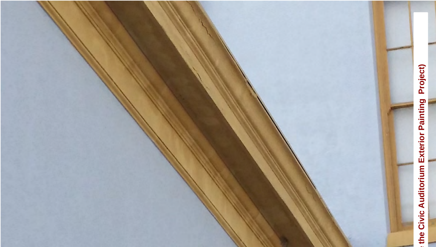
Plaster & wood overhang and crown showing water staining due to caulking failure NE corner of building
