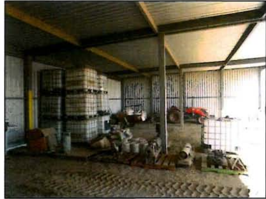
Interior view of the equipment shelter.
