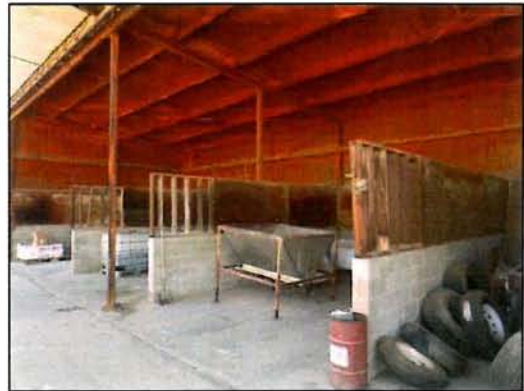
Interior view of the product storage shelter.
